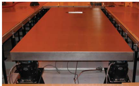
STACIS® System on “risers” installed as a custom designed TMC Quiet Island® subfloor platform to support an eBeam lithography tool in a 36 in. tall raised floor.
